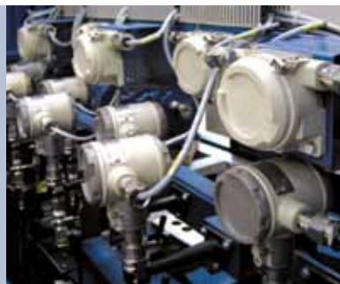
Pressure and temperature transmitter for monitoring argon compressors
