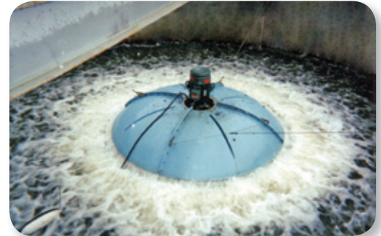
Aqua-Jet II® Aerator in operation.
